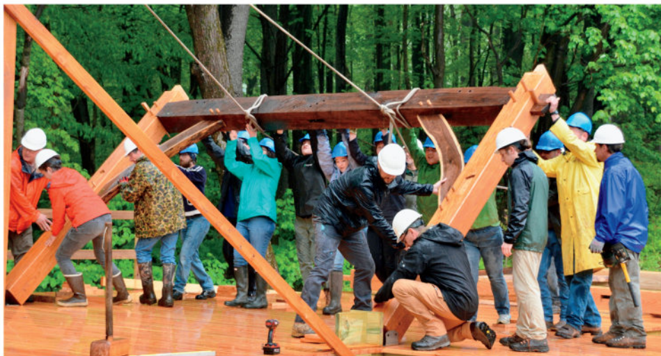
Careful coordination between volunteers lifting timbers and pulling ropes was needed to raise the assembled bents into place. Photo by Leo Glenn.
